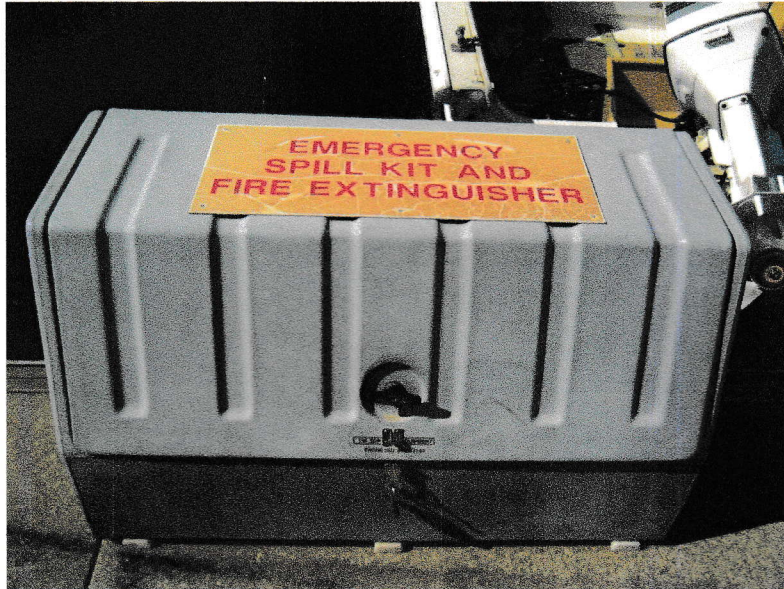
FUEL WHARF SPILL KIT WITH CONTAINMENT BOOM AND FOAM FIRE EXTINGUISHER
