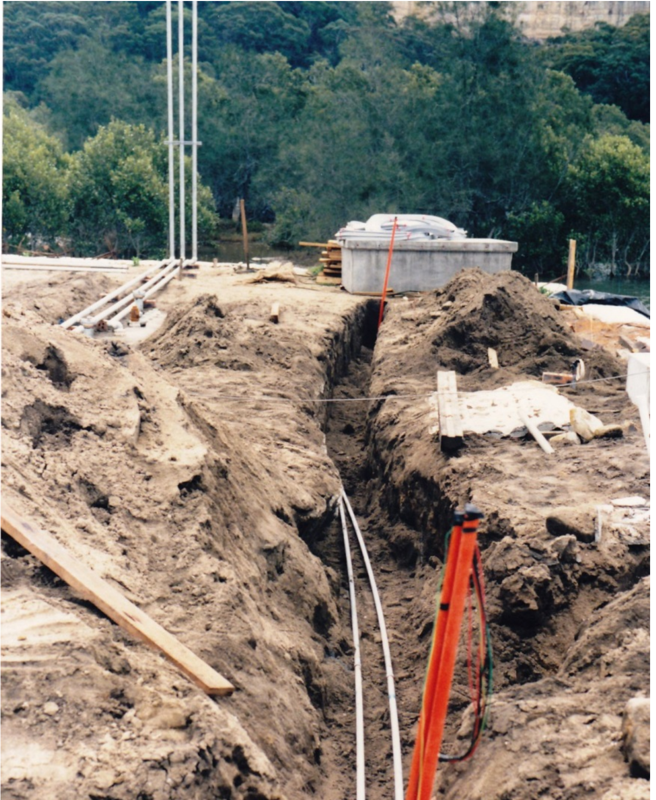
THREE FUEL VENT PIPES. VIEW LOOKING TO THE WEST. ON THE RIGHT IS SANDBROOK INLET
